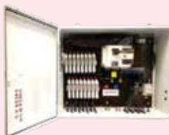
String Combiner Box
